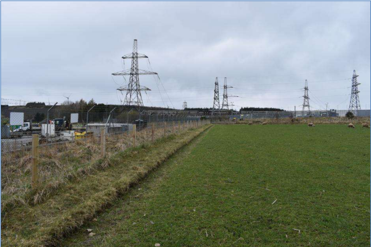
Plate 3: View southwest towards Blackhillock Substation ( Asset 83 ), from southwest side of Site
